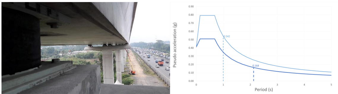
Figure 9: View of the LRB isolation level, between the precasted piers heads and the U shaped viaducts and the Response Spectrum of a span with and without isolation system
